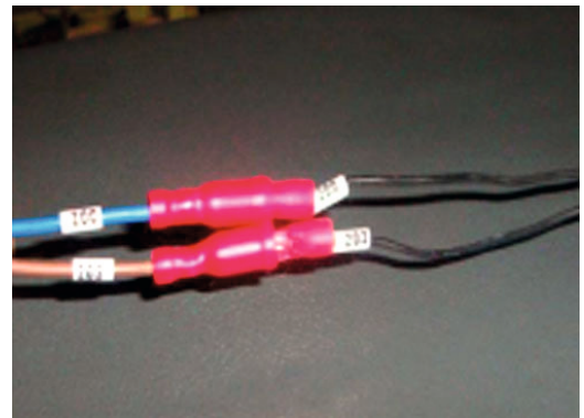
Picture 12 (end switch connection)
